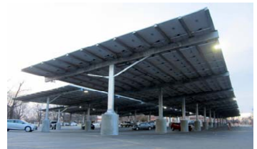
Meridian 321.55 kW Project : Veterans Hospital Fayetteville, AR
